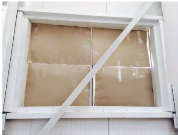
Figure 22 North-facing skylights are blocked with chipboards
