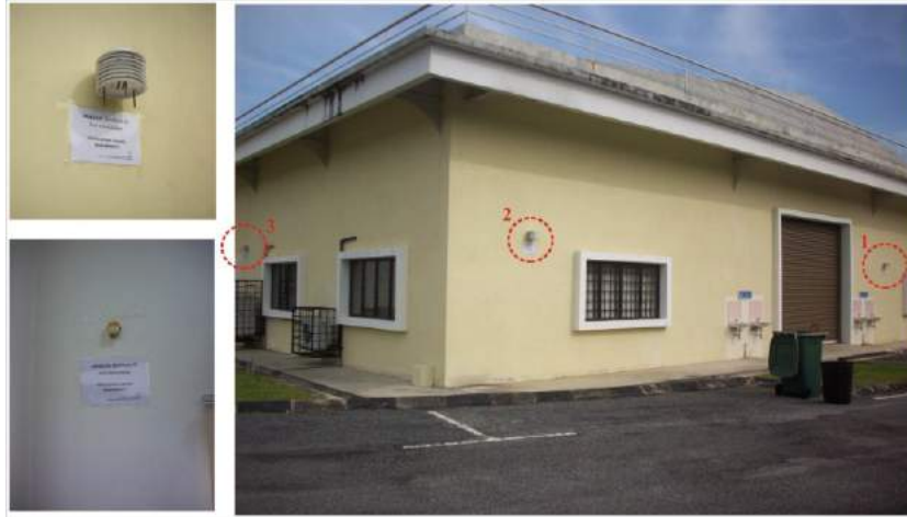
Figure 4.61 Example installation of Tinytag at outdoor and indoor wall
